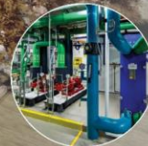
ROBUST HVAC FOR ENERGY PERFORMANCE
